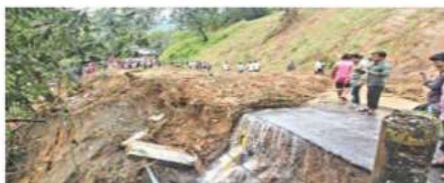
Figure 7a Hills damaged by landslide
